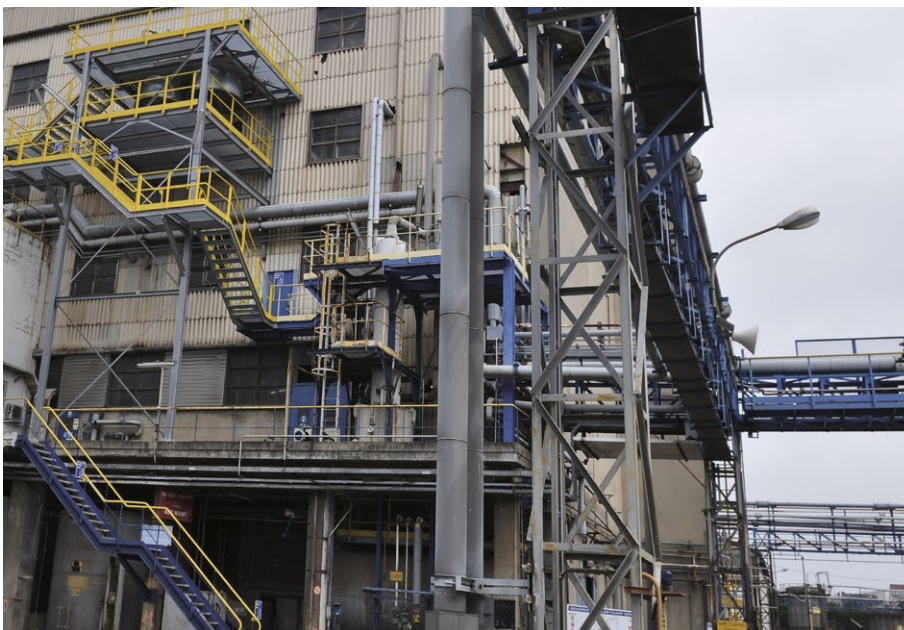
Figure 1: In the Vallée de la Chimie to the south of Lyon (France) a new plant for recovering rare earths from the luminescent powder used in energy-saving and fluorescent lamps has been erected next to the vanillin production line
