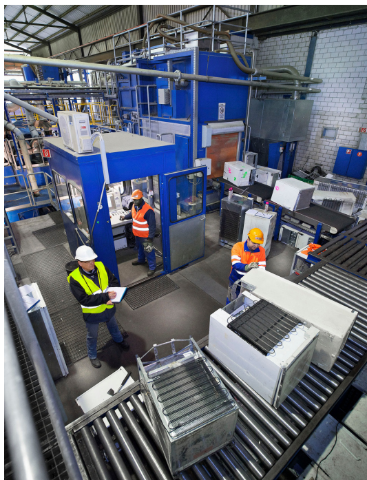
A look into a refrigerator treatment system
